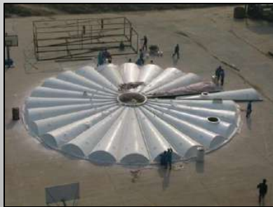
60' dia. hot clarifier covers for FLS/SNC Lavalin Ambatovy
